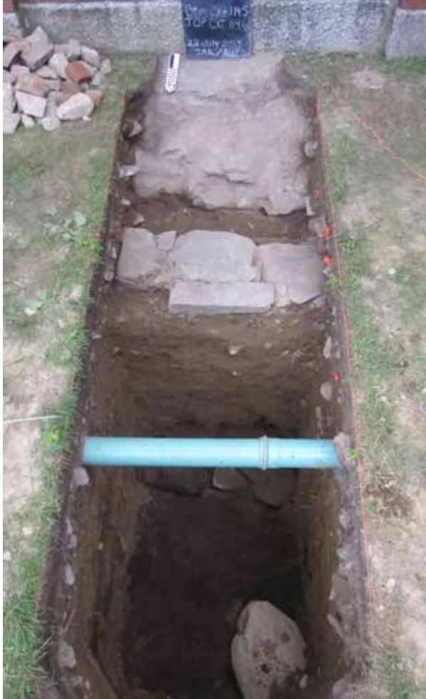
Figure 28. Door footer in EU206, north of a later concrete cap placed for foundation repair.
