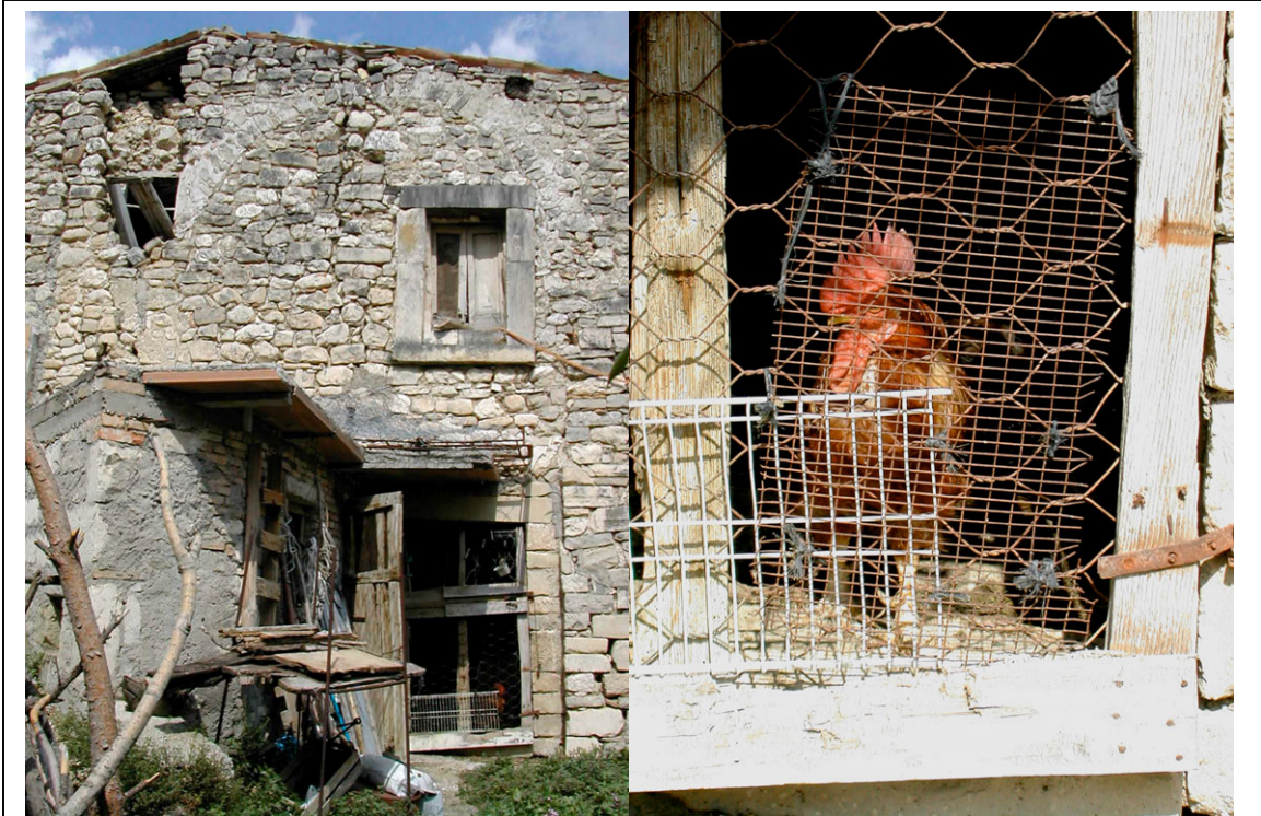
Figure 3.4: A new animal resident in a house abandoned by its former human occupants, located in the lower, slide-damaged quarter of Taranta Peligna. When I walked up to this stone house, which is beginning to split down the middle (see crack from roof through embedded arch to main door), I was surprised to discover that it had been turned into a rather grand if dilapidated chicken coop. The rooster (in the lower, right-hand corner of the door opening in the photo at left) stares back through a gate made of various improvised materials. The practice of using old structures as animal pens is actually quite common – and is probably connected to the tradition of incorporating animal stalls into the lower levels of houses (for the efficient protection of both the animals and humans under one roof, with added benefit of additional body heat in winter); animals were still commonly quartered in Aventino Valley villages until the mid-twentieth century.
