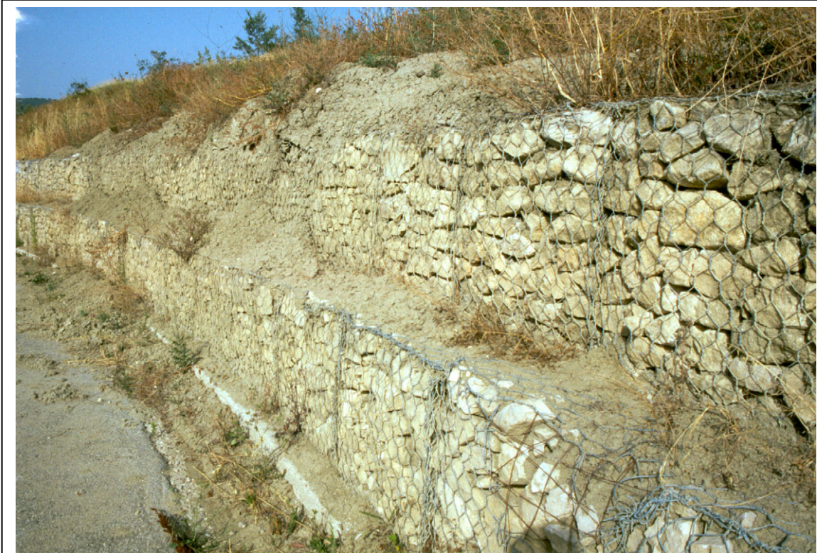
Figure 7.22: View along the road toward Colledimacine of the remains of a recent mudslide (most of which was bulldozed away after it had flowed into the roadway) piled on the ledges of a reinforcing wall made of stacked metal cages of stone.
