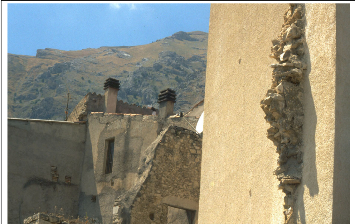
Figure 6.17: View of partially destroyed walls and wall sections protruding from still standing buildings in Lama with the Majella in the background.
