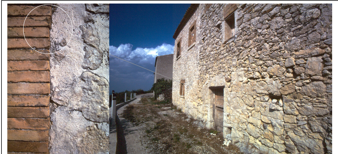
Figure 8.32: Close-up and perspective views of a boundary between houses in western Colledimacine.
