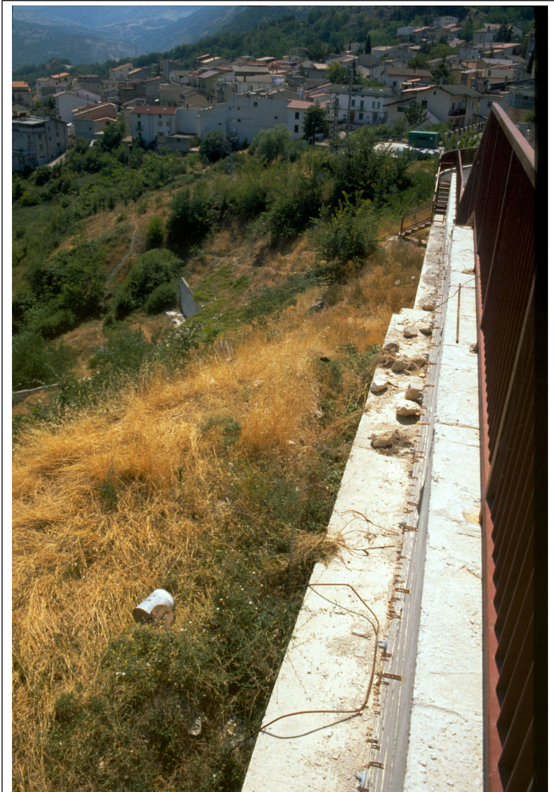
Figure A.11: Cement retaining walls temporarily separating an area subject to frequent landslides from the rest of Lama. (See also bottom image in figure 6.30)
