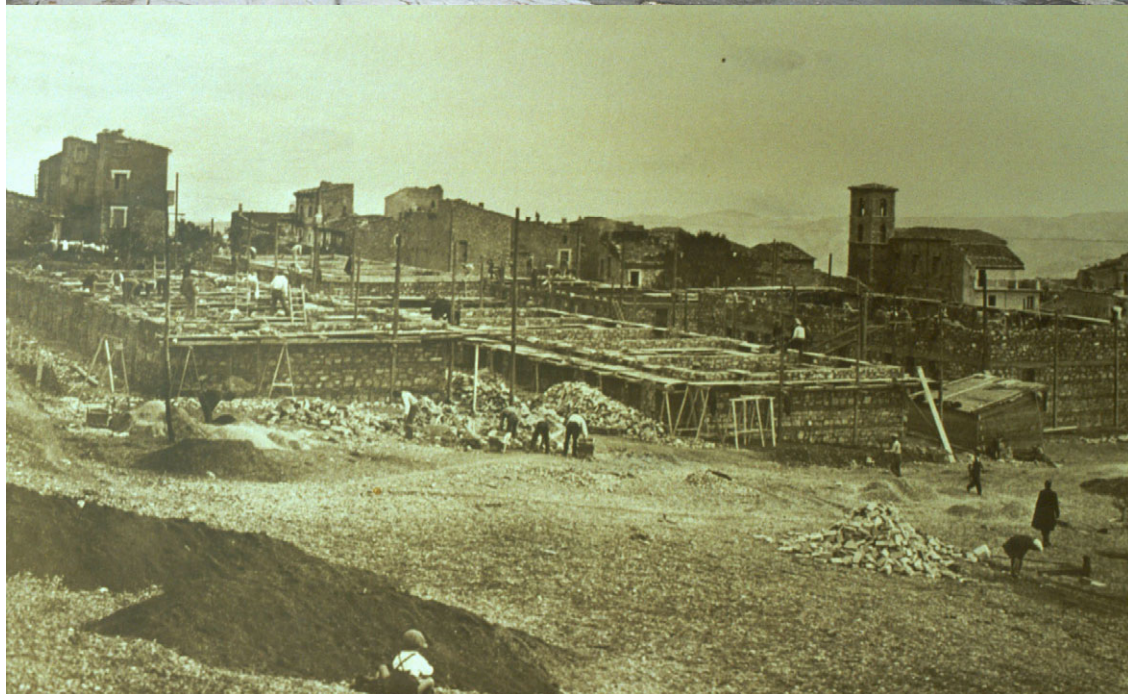
Figure A.16: Two views of Lama: below is a photograph of buildings under construction, soon to become housing for the homeless due to the 1933 earthquake (Lama municipal archives); above is a close-up shot of the buildings in 2001. (See also figure 6.33)
