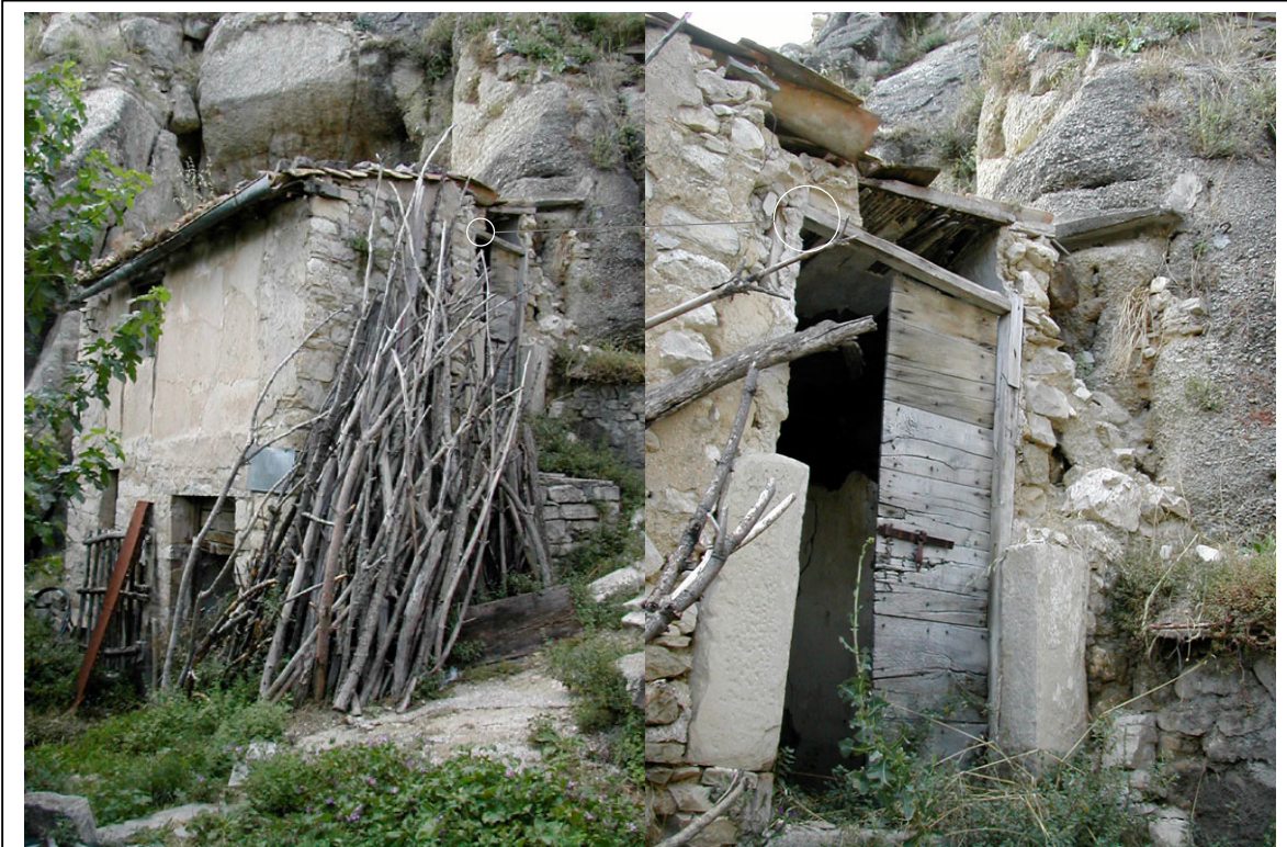
Figure 7.9: A small rural structure at the base of Taranta Peligna, built mainly from materials found nearby, which uses the cliff behind it as the main support for a makeshift back wall. While the large vertical stack of branches suggests continued use, inside a collapsing roof, rotting strands of braided garlic, bird droppings, and trash indicate abandonment within the last five to ten years. When this house eventually collapses, little will remain as evidence of its former existence apart from metal artifacts and a pile of stone interspersed with fragments of terracotta roof tiles.
