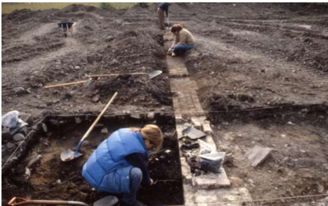
Figure 2. Photograph of MAAH excavations onsite. An archaeologist reveals the footings of the west wall of the car shop.
