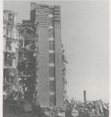
As Columbia Point buildings come down, above, the $190 million Harbor Point (top photo) will rise.
